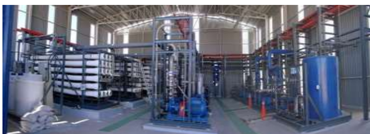
Figura 1: Planta de osmosis reversa, Codelco (Chile).
