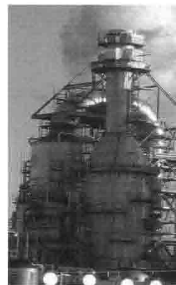
FCCU Regen Gas 620 MMSCFD
