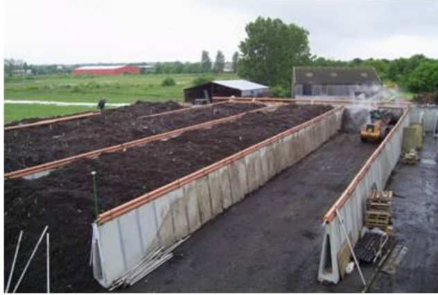
Photograph 4.14: Open Aerated Bays
